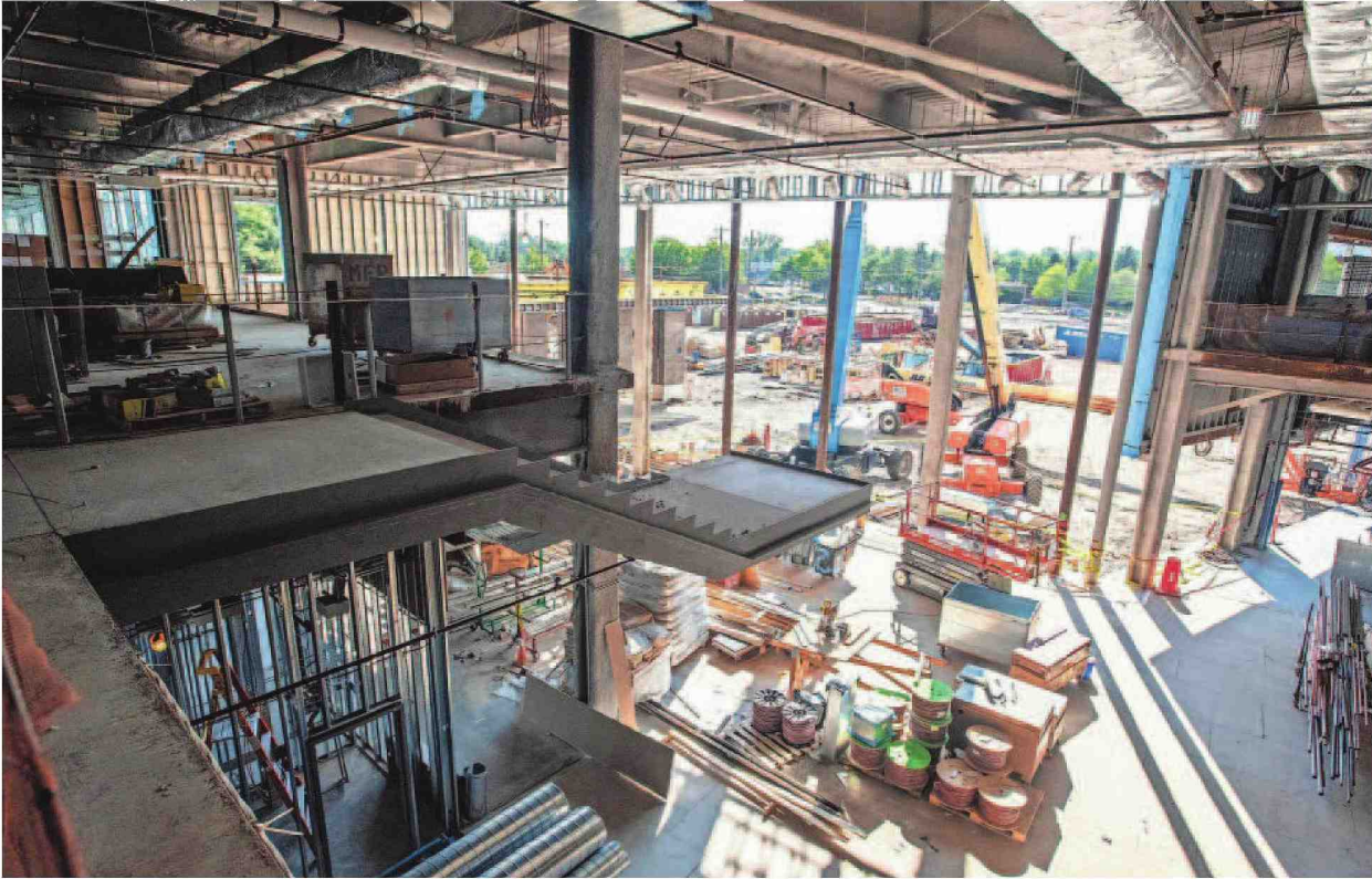
Construction on the lobby of the new Valley Hospital in Paramus is seen on Tuesday. Dedicated elevators will carry visitors to the patient floors, while others, activated only by ID badges, will be for staff use.
