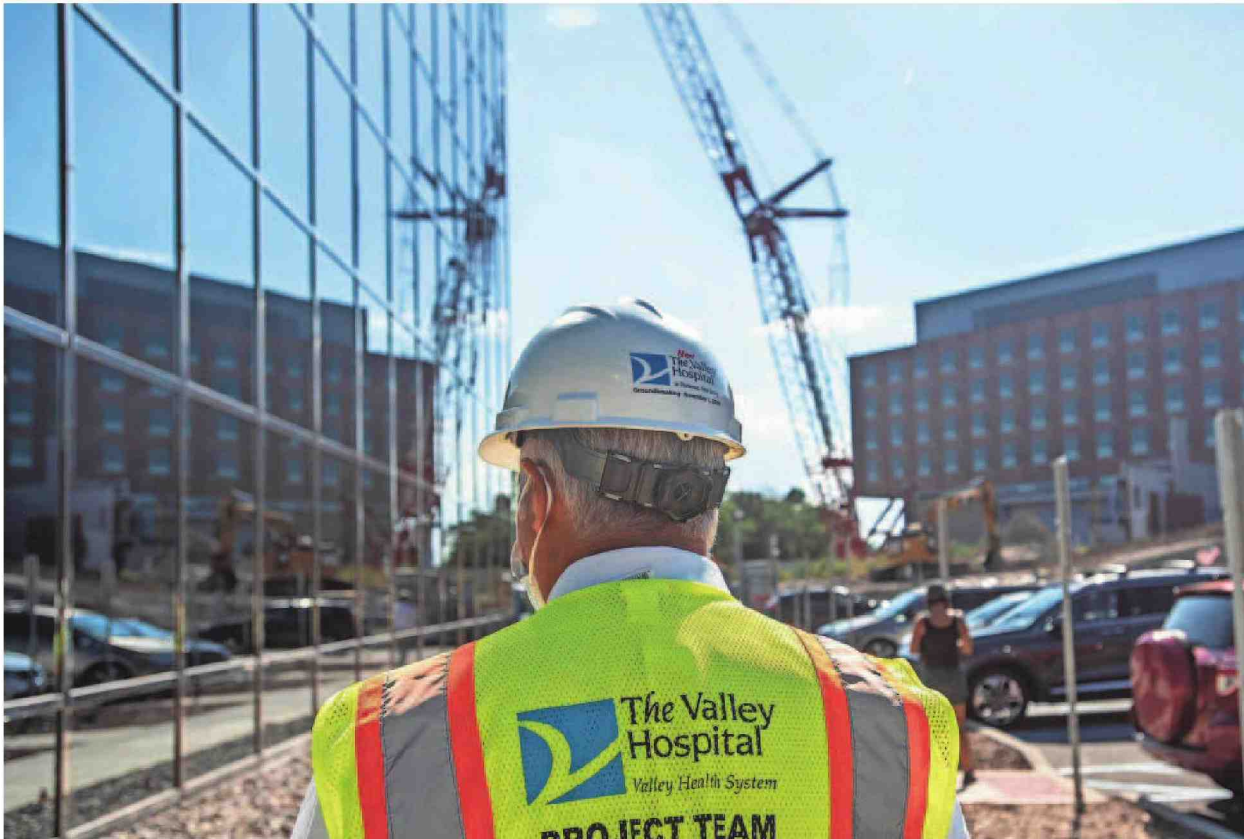
Joseph Lorino, the vice president of facilities management for Valley Health System, leads a tour of the new Valley Hospital in Paramus. Lorino walks along the building site, currently populated by more than 500 construction workers. PHOTOS BY ANNE-MARIE CARUSO/NORTHJERSEY.COM
