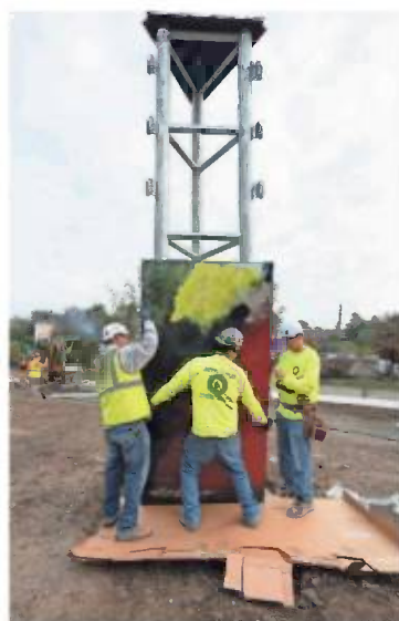
Carpenters for Edward Leske Company put up the panels of the mural in the courtyard of the new Valley Hospital in Paramus on Wednesday.
